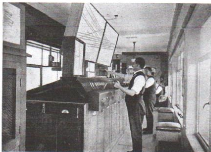
Fig. 1. Interior of Franklin-street Junction Special Signal Cabin
