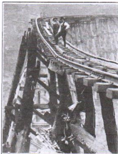
This picture shows in a graphic manner the damage done by bush fires to one of the trestle bridges on the line from Warragul to Noojee. Five of the seven bridges were damaged, but work is already proceeding on their reconstruction.
