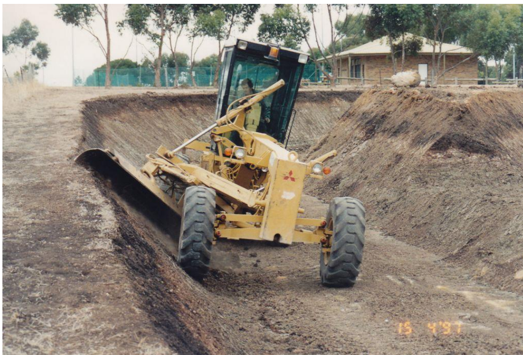
Earthworks being undertaken to build the Bulla Hill Railway during 1997.- (Pic: FB TLSS)
