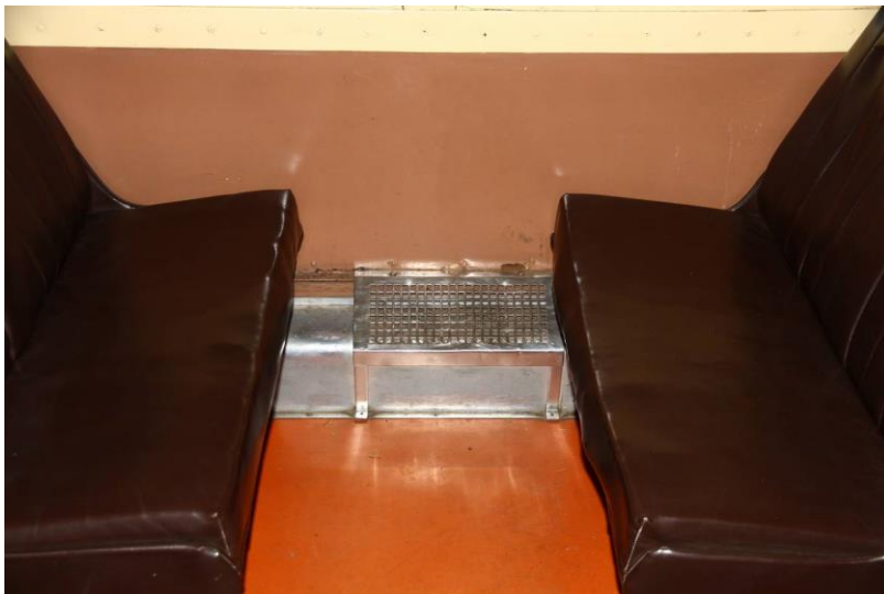
The heaters under the windows on both sides of the rail car
