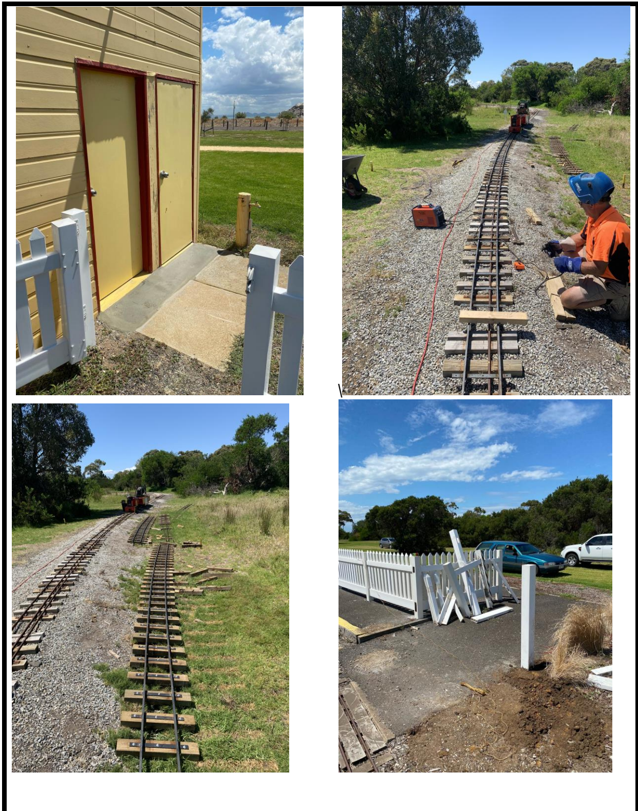
Pictures from our recent February Working Bees showing the new Signal Box Ramp, new Culvert Bridge Curve trackwork & Platform No.2 fencing re-arrangement. Thanks go to our small but loyal team – well done to all . (Pics Neil Hester & Brian Coleman)
