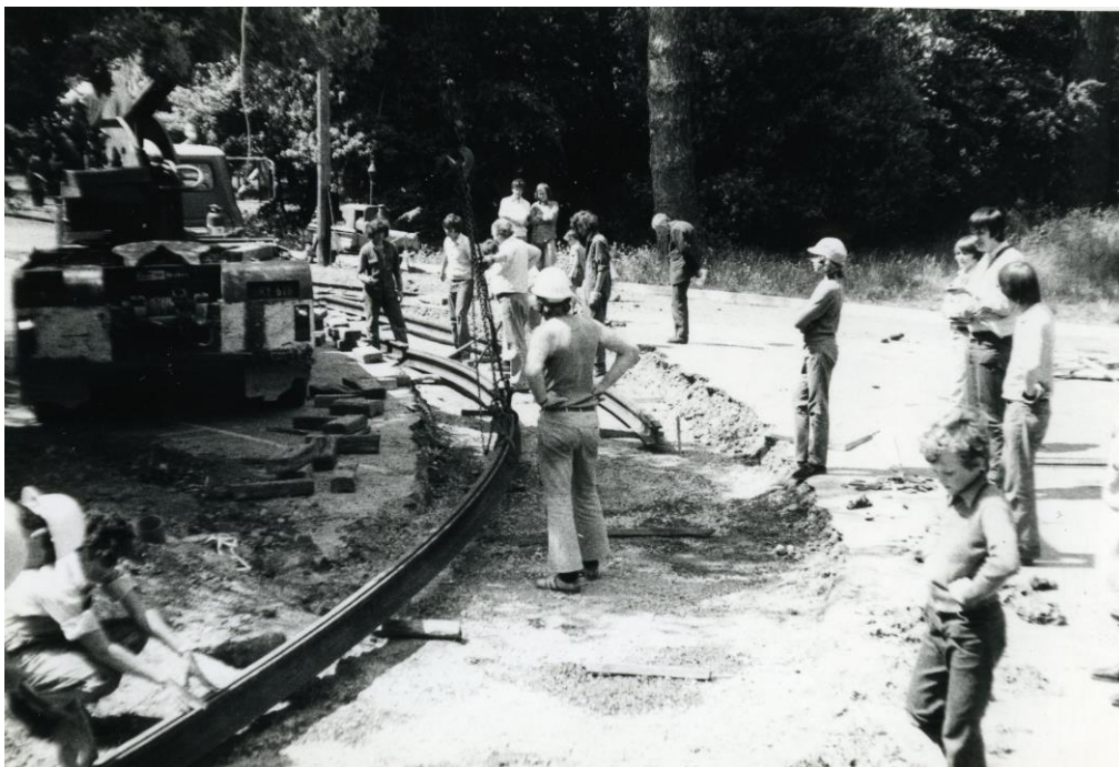
Laying the tracks to access the depot from Wendouree Parade in late November 1974, when things were done largely manually. All volunteers except the mobile crane crew. (Pic: Clyde Croft)
