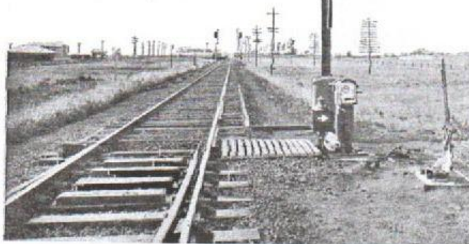
Electric switch lock on siding points
